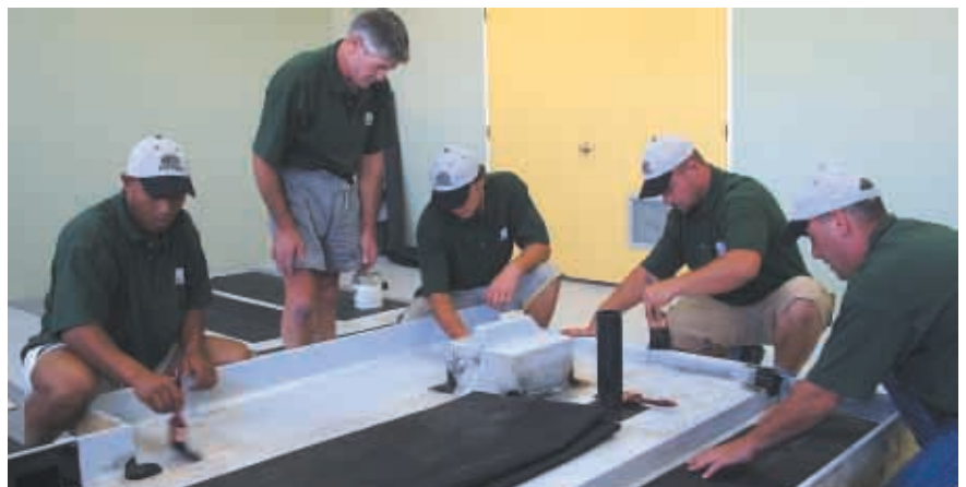
A training session in progress at the Ardex purpose built National training facility in Christchurch
