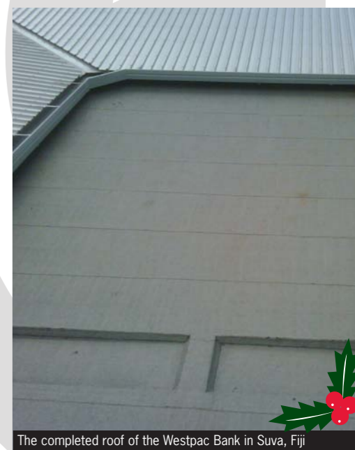
The Westpac Bank in Suva has been re-roofed in Shelterbit Mineral Torch On Membrane.
